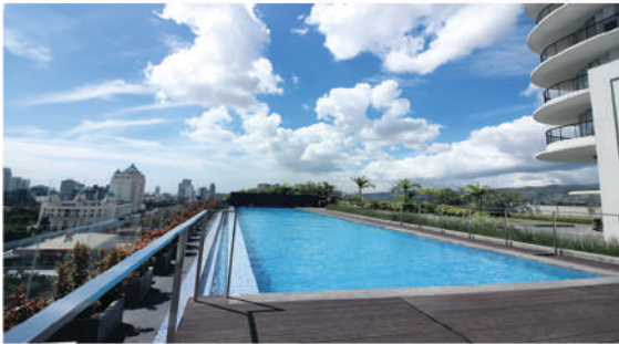
CALYX RESIDENCES - Swimming Pool @ 10/F , I.T. Park, Lahug, Cebu City Re-waterproofing works - Torch-applied membrane waterproofing removed and applied with CWS100
