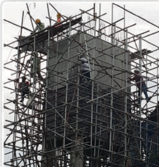
PEACEVALLEY SUBD. WATER TANK, CEBU CITY
